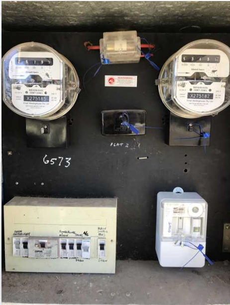
No safety switch identified in meter box.
