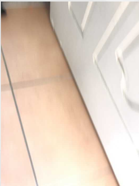
Minor weather damage to entrance door.
