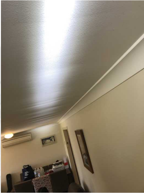
Minor age related sagging observed to plasterboard ceilings.
