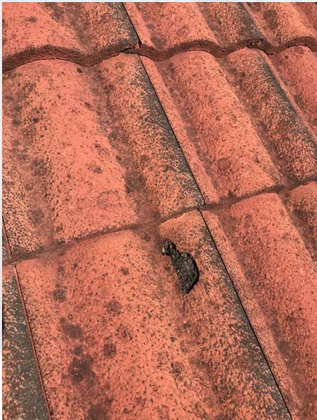
A deteriorated tile identified above entry. A few chipped tiles identified.
