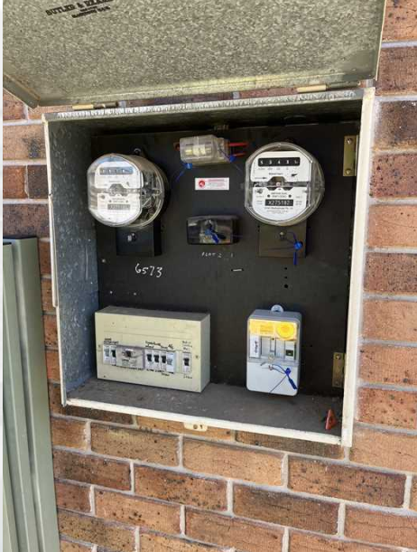
Meter box, No durable notice to indicate any recent termite treatment or post construction management system installed
