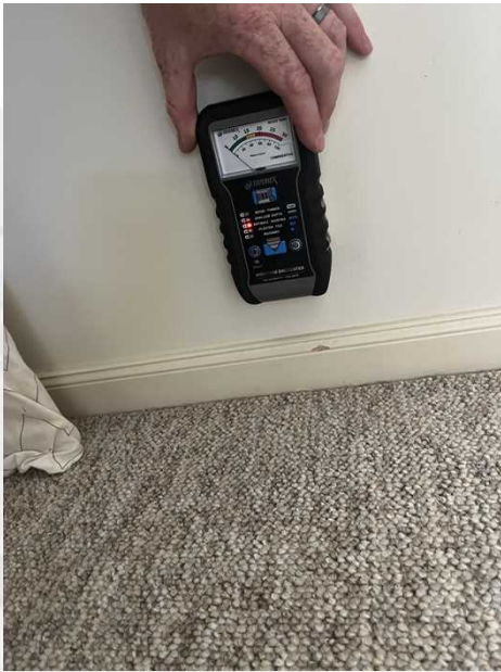
All accessible internal dry walls, Tramex moisture meter observed no high moisture readings at the time of inspection.
