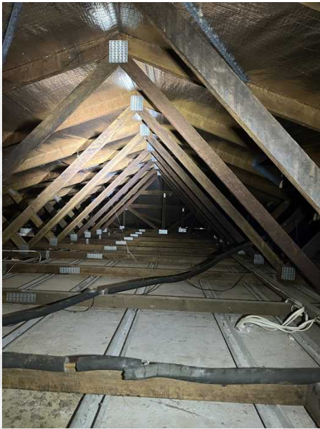
The roof void was inspected, no visible evidence of timber pest activity at the time of inspection
