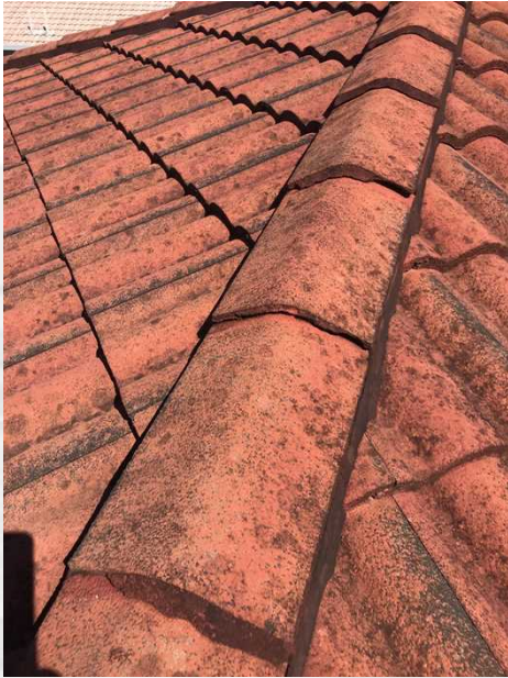
Cracking to the pointing of capping tiles observed.
