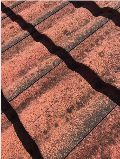
Couple of cracked tiles identified requiring replacement.
